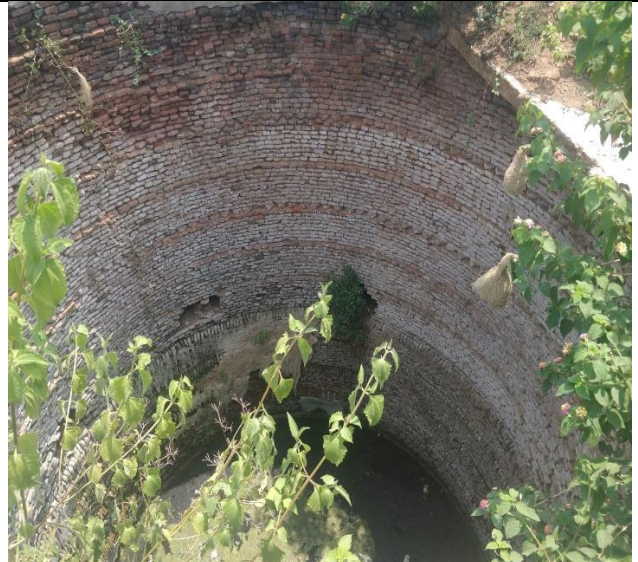
Open well present at the site
